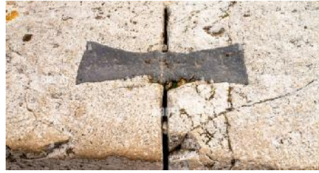
Figure 9: Stone joined by iron pegs fixed as “X” joint. (Source: Parmar S. P., Insights of Modhera Sun Temple [27])
